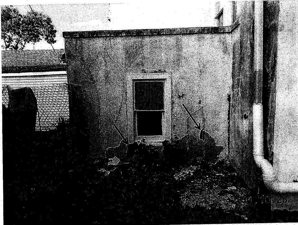
PHOTO NO. 1.19: Priority Repair 5 – Spalled plaster with wire lathe façade over rotting timber wall framing – East Elevation, Grid H-I: El. 6' +/-
