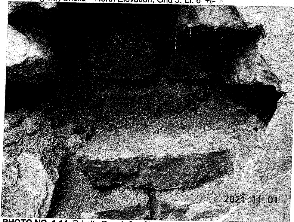
PHOTO NO. 1.14: Priority Repair 2 – Close-up view of severely damaged brick masonry piers. Note: condition of interior wythe bricks and mortar – North Elevation, Grid 5: El. 6' +/-
