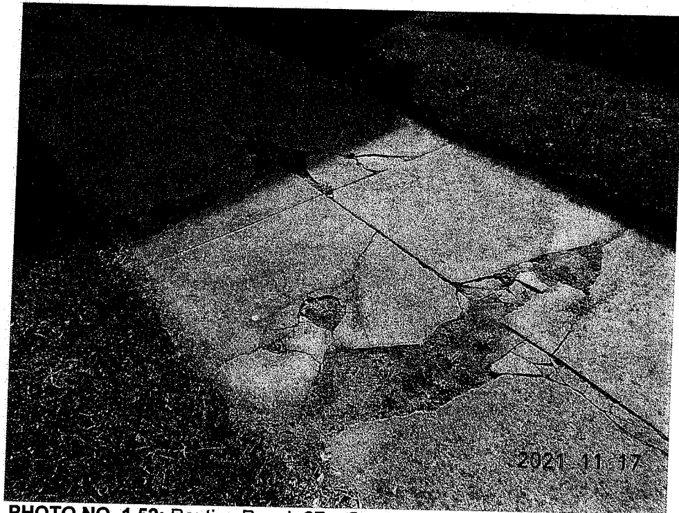
PHOTO NO. 1.52: Routine Repair 27 – Cracked and spalled concrete sidewalk – Site, Grid F-G/6-8
