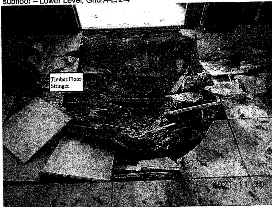
PHOTO NO. 1.24: Priority Repair 7 – Overall view of Fellowship Hall with failing floor system due to severely deteriorated timber stringers and subfloor – Lower Level, Grid A-E/2-4
