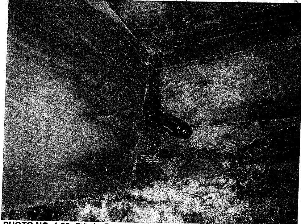
PHOTO NO. 1.22: Priority Repair 6 – Rotting and soft timber floor beam at bearing ends due to active water infiltration – Sanctuary Framing, Grid A/6-7
