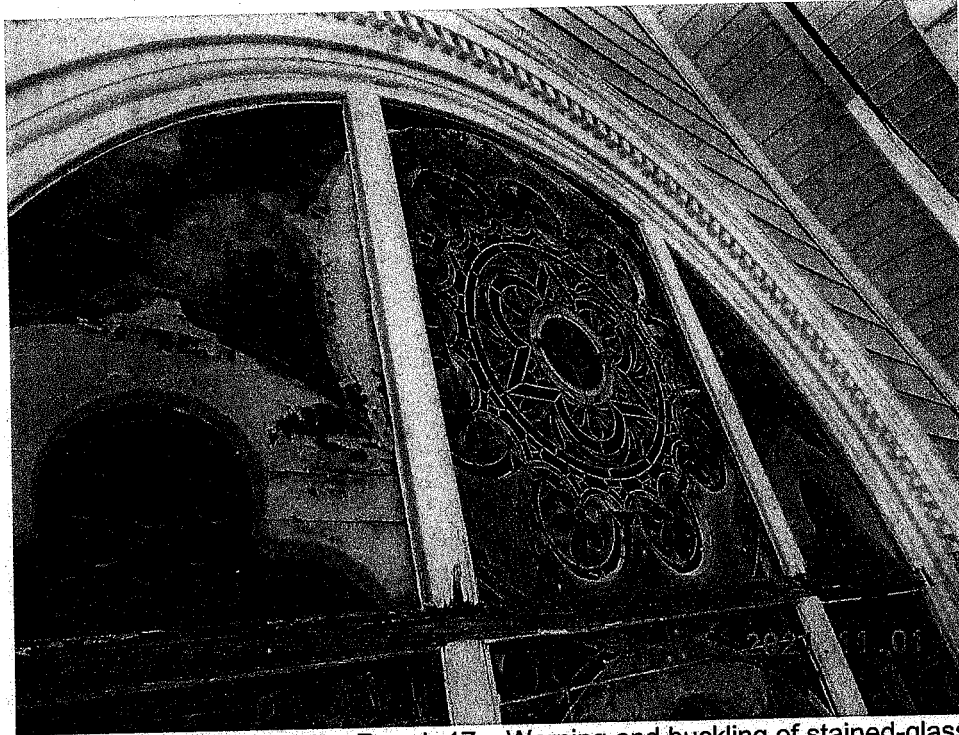
PHOTO NO. 1.42: Routine Repair 17 – Warping and buckling of stained-glass window with deteriorated timber frame – North Elevation, Grid 5-6: Ht. 25'
