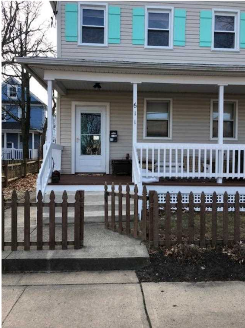
5 5-IMG_3373 611 Park Place Porch 6" 1" from sidewalk excluding stairs
